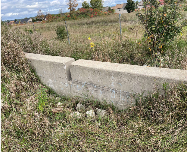
125 mm wide rectangular contracted weir on the SWM Outlet Control Structure
