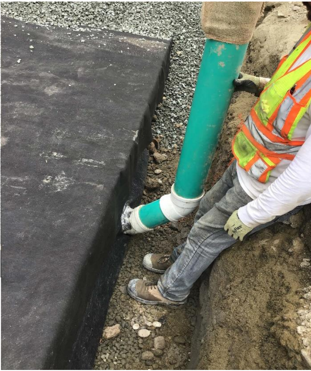
FIG#1: INSPECTION/ VENT PORTS
