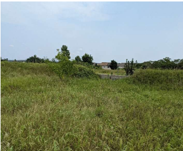
Trapezoidal sharp-edge weir on the SWM Outlet Control Structure
