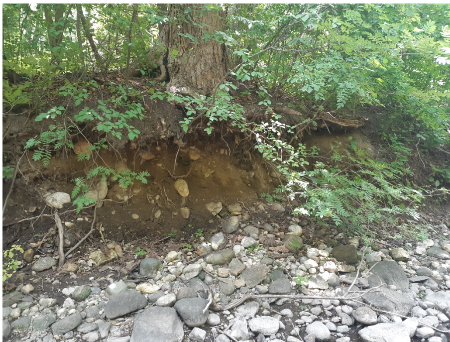
Photo 2 Signs of erosion on channel banks, June 2021.
