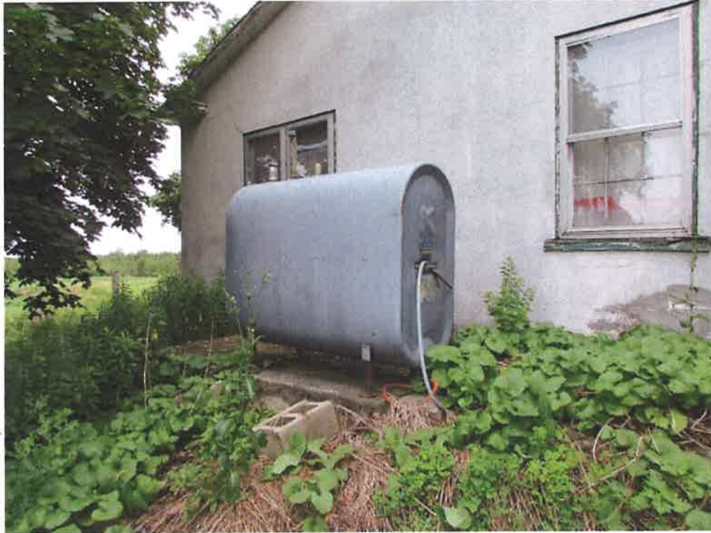
View of the heating fuel oil aboveground storage tank on the west side of the residential building.
