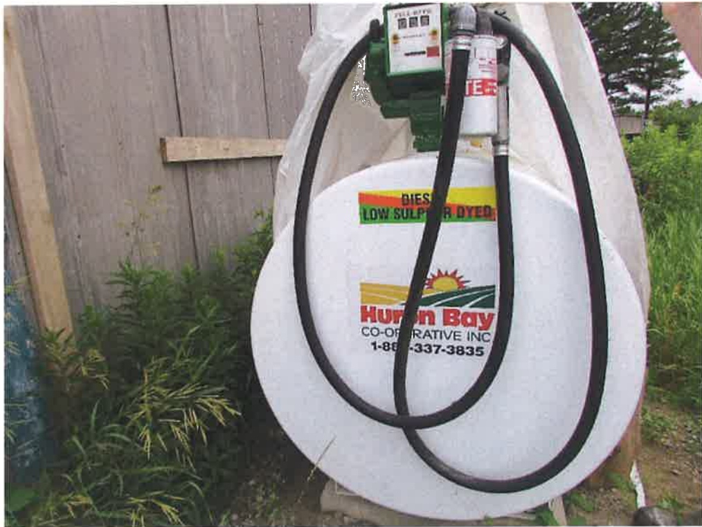
View of the diesel aboveground storage tank on the north side of the tractor storage shed.
