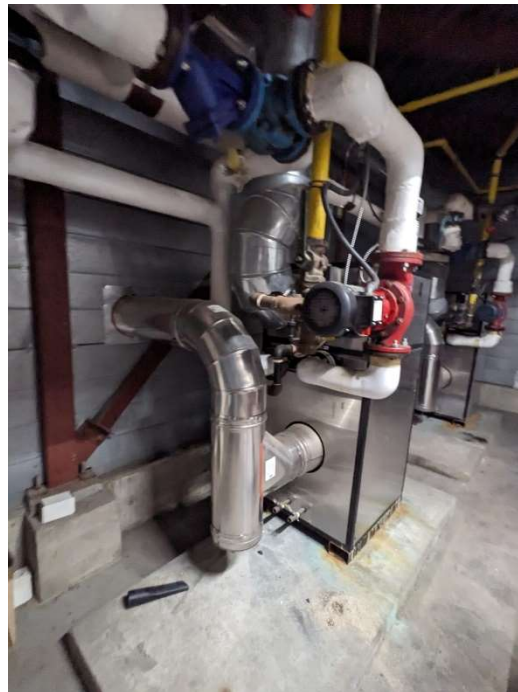
18. View of the boilers on the 2 nd floor of the building, facing south
