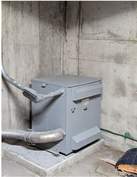
15. One transformer in the basement, facing northwest
