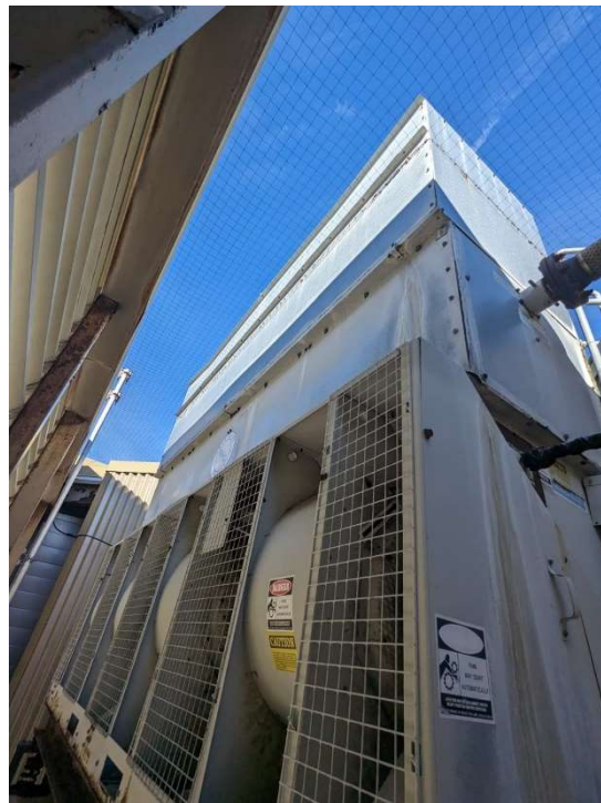
20. View of the cooling tower on the top of the roof, facing south
