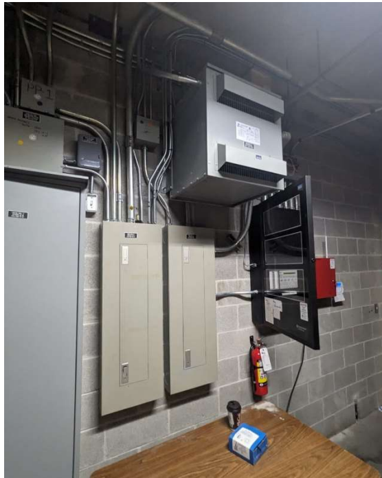
16. The other transformer in the basement, facing west
