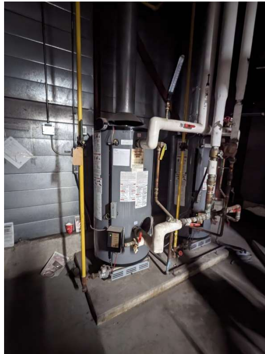
19. View of the hot water tanks on the 2nd floor of the building, facing east
