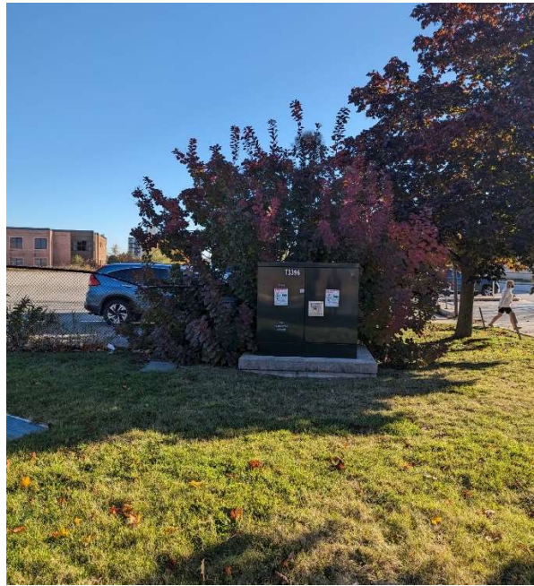
5. Transformer T3396 adjacent to the Phase One Property, facing east
