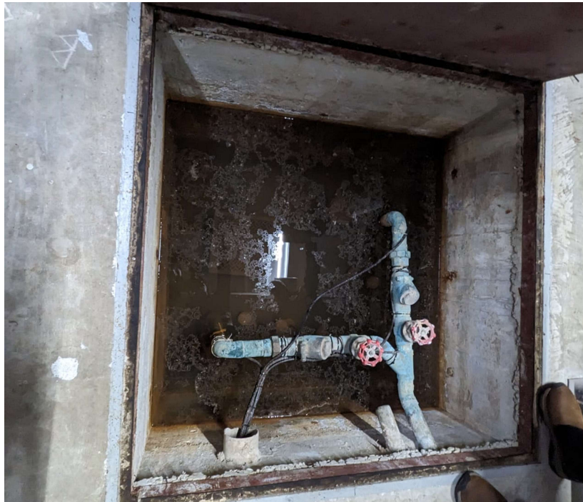
13. One sump pit in the basement, facing the ground
