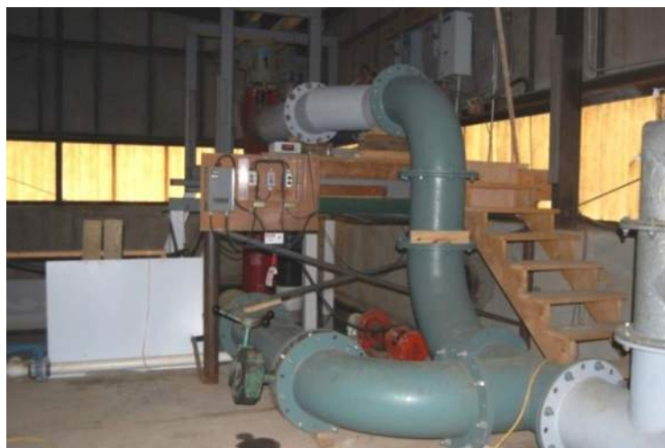
Figure 5: Photograph Showing Laboratory Pumps
