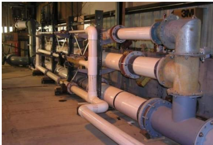
Figure 4: Photograph Showing Laboratory Flow Meters
