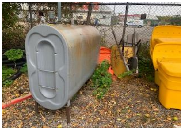
Picture 10: View of the former 910L fuel oil AST, located south of Site Building B, facing east.
