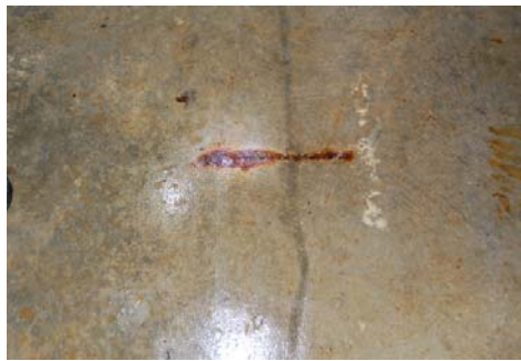
Rebar Exposed on the Floor
