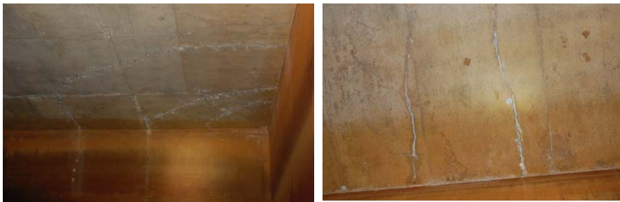
Previously repaired cracks on the soffit
