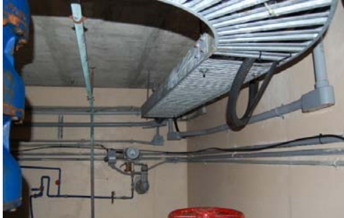
Cable Tray and Conduit at Lower Level
