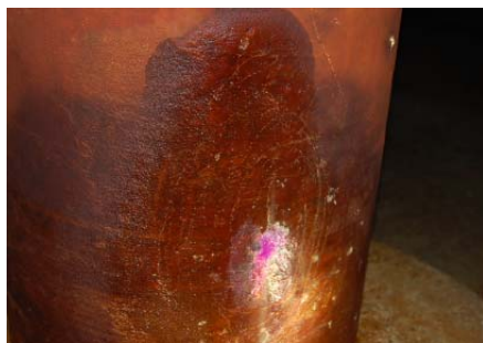
Column C1: soft spot near bottom
