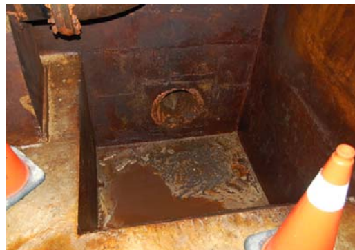
Intak and Drain pipe connections inside Cell No. 1
