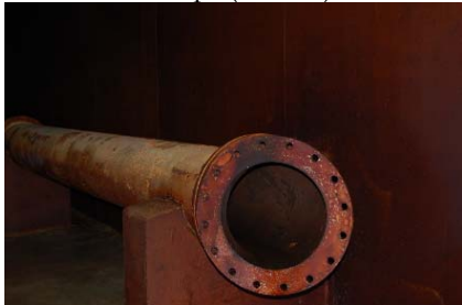
End of Feed Pipe (400mm) in Cell No.2
