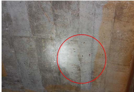
Exposed reinforcement (Roof)
