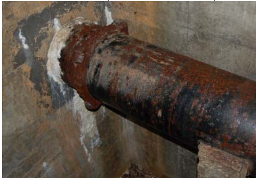
Intake pipe penetrate reservoir wall
