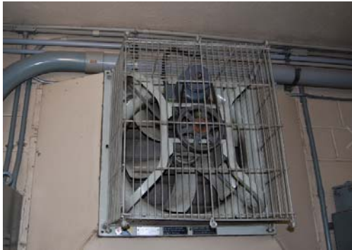
Wall Mount Ventilation
