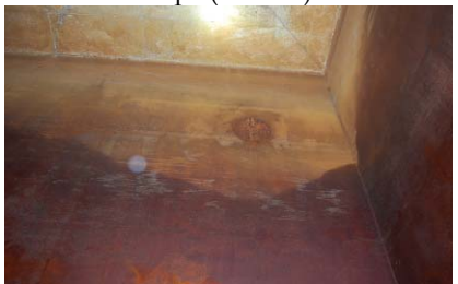
Overflow Connection in Cell No.1
