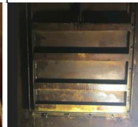
Sluice Gate Between Rsvr Cells
