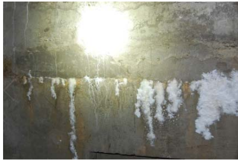
Calcium deposition on the wall
