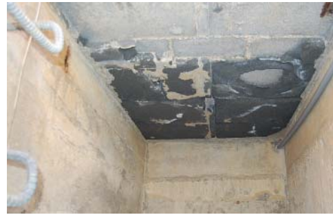
Flaking off ceiling insulation
