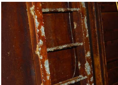
Aluminum Ladder in Cell No.2
