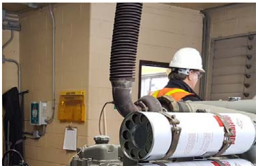
Diesel Combustion Exhaust
