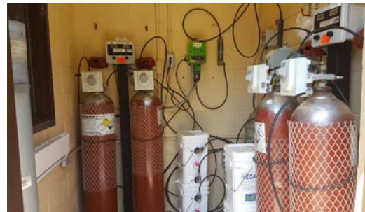
Gas Chlorination System
