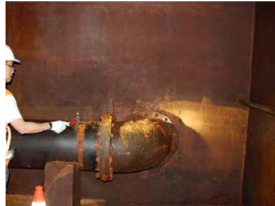
Intake Pipe (400mm) in Cell No.1
