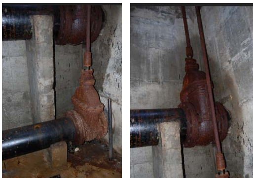
Intake Gate Valves (300mm and 400mm)
