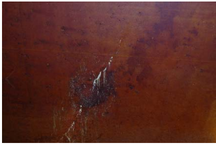
Typical cracks on the internal wall
