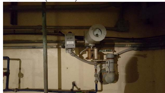
Reservoir Level - Pressure Type (LIT-2110A)
