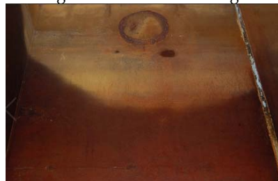
Overflow Connection in Cell No.2
