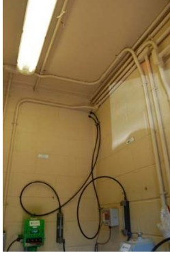
Chlorination Room - Interior
