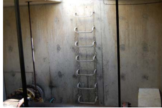
Access to Valve Chamber
