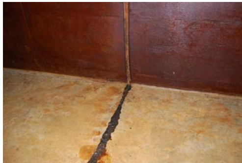
Expansion Joint Sealant (Floor and Wall)
