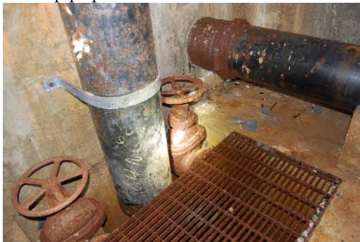
Overflow pipe and two Drain Valves
