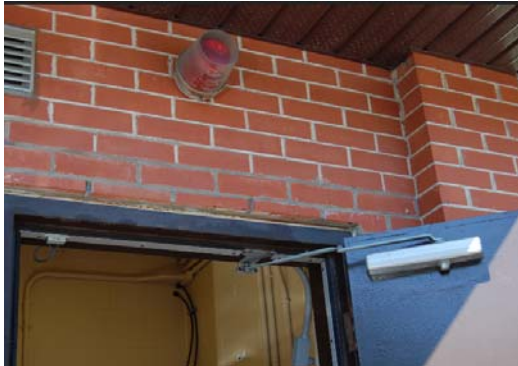
Chlorine Gas Alarm Strobe Light
