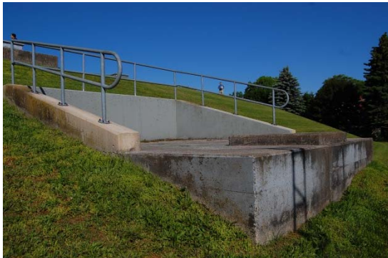
Exterior - Inlet Valve Chamber
