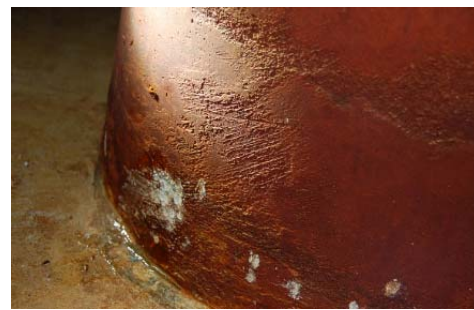
Column C2: soft spot near bottom
