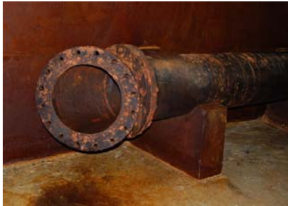
End of Intake Pipe (400mm) in Cell No.1
