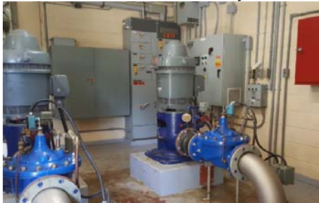
Vertical Turbine Motor and Pump Control Valves
