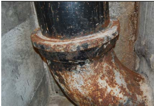
Overflow pipe from the reservoir cell
