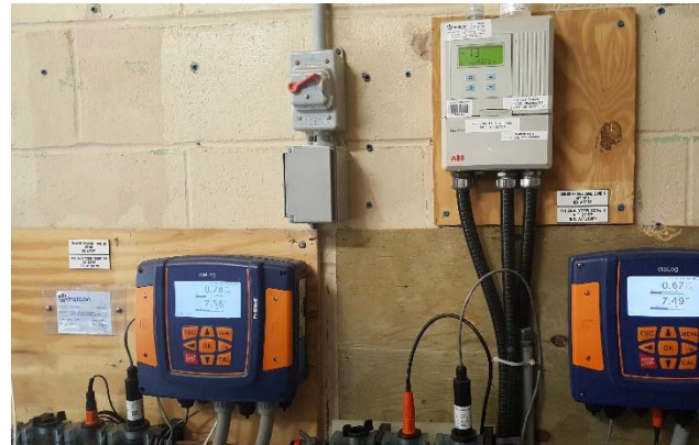
Zone 1 and 2N Chlorine Analyzer (AIT-2113, AIT-2119); Zone 1 Flow (FIT-2111)
