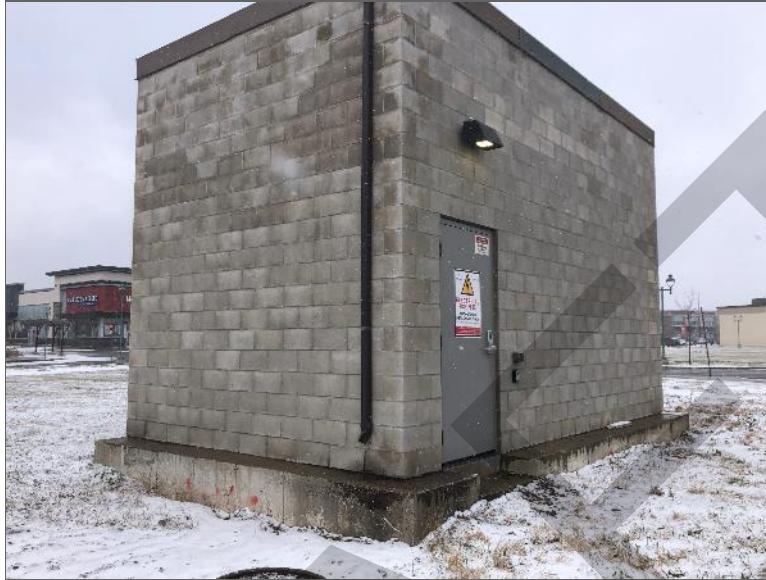
Photo 13 – Hydro vault located in the central portion of the Phase One Property, looking northwest.
