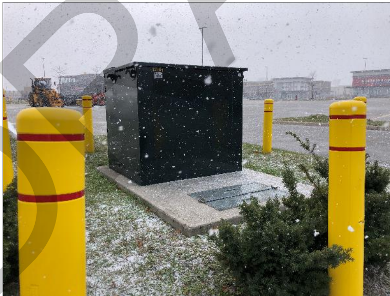
Photo 12 – Pad-mounted oil-cooled electrical transformer located in the northeastern portion of the Phase One Property, looking south.
