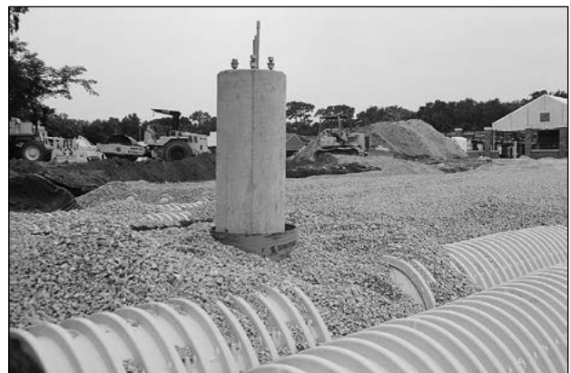
Figure 15 – Chamber bed placed around light post.
