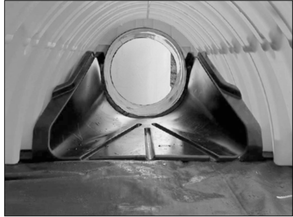
Looking down the Isolator Row PLUS
