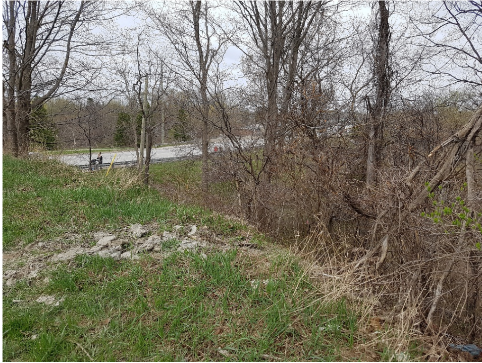
Photograph 1: Steepest portion of slope (about 1H to 1V) adjacent Big Bay Point Road.
