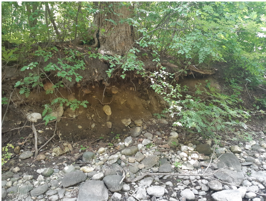
Photo 2 Signs of erosion on channel banks, June 2021.
