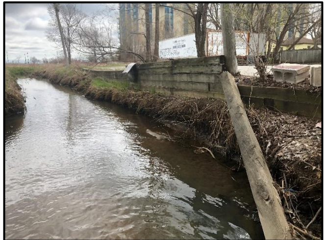
Photograph 8. (Photo Location 7) Downstream view of existing wooden retaining wall along southern channel bank (off property). Note: undermining of retaining wall and leaning hydro poles observed
