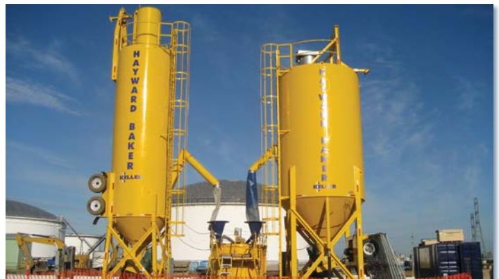
A soil mixing grout slurry batch plant. Real-time monitoring of all mixing parameters allows for control of batching and pumping operations.
