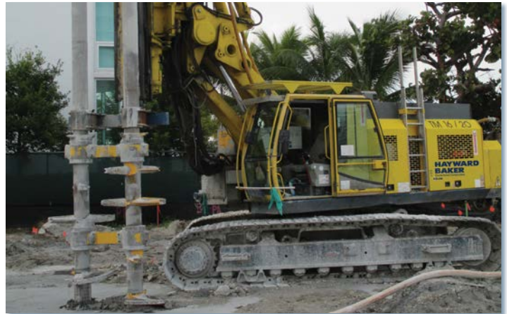
Dual axis wet soil mixing rig used to construct a perimeter retaining wall prior to excavation for a planned high-rise in Florida.
