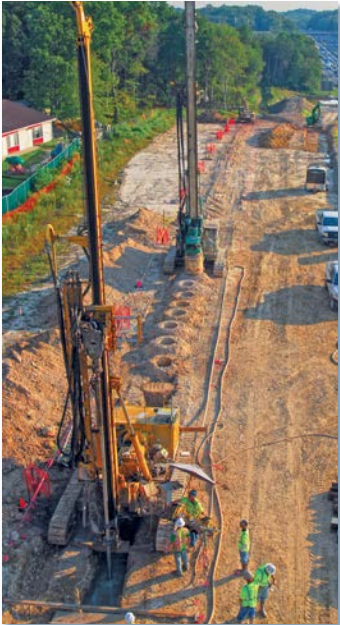
Above: Soil mix columns constructed along the alignment of an existing waterline provided a containment system to protect the critical utility in Maryland.
