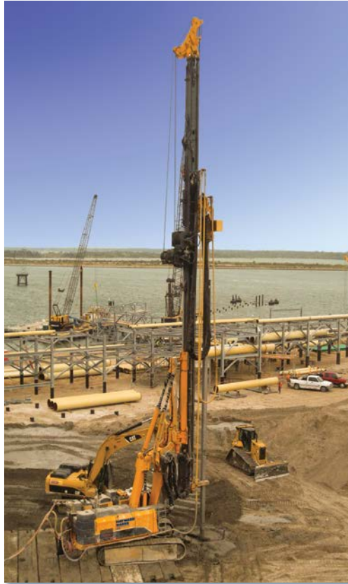
Soil mixing performed to increase bearing capacity and reduce settlement for planned tanks in Texas.
