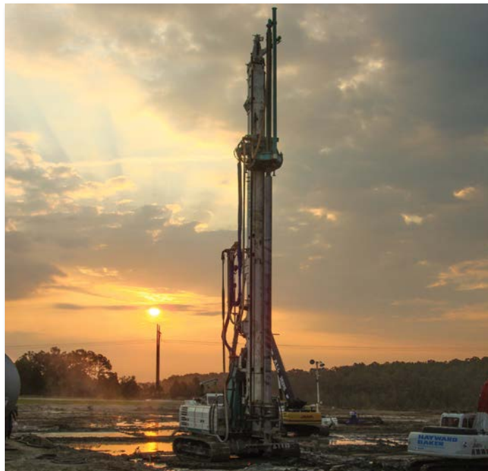
Soil mix columns constructed for foundation support and liquefaction mitigation for the expansion of a nuclear plant in North Carolina.
