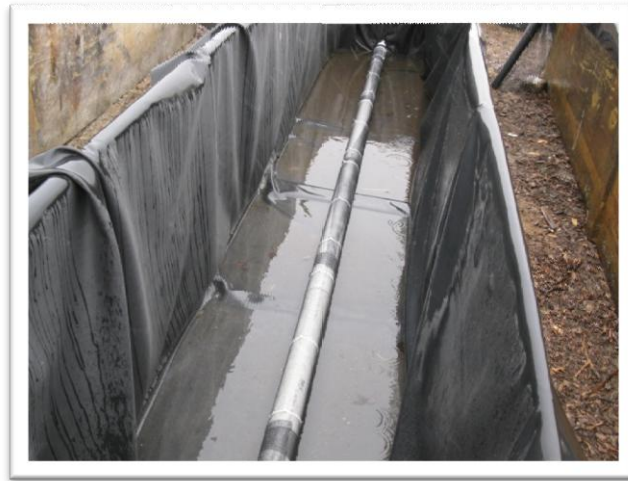
Figure 2-2 Fibreglass reinforced plywood trough lined with pond liner with 3 inch PVC underdrain pipe running the length of the bioretention cell
