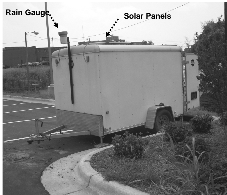
Figure 3. View of the Mobile Monitoring Unit (MMU) installed at the Mitchell Community College testing site.
