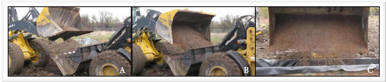
Figure 2-4 Mixing of bioretention soil between the buckets of two front end loaders and dumping of soil mix into the cell
