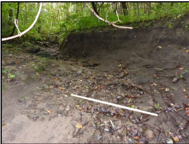
Photo 23 (Photo Location 25) Reach BEA2-7 Downstream view of bank erosion. Note: minimal flow present within channel.
