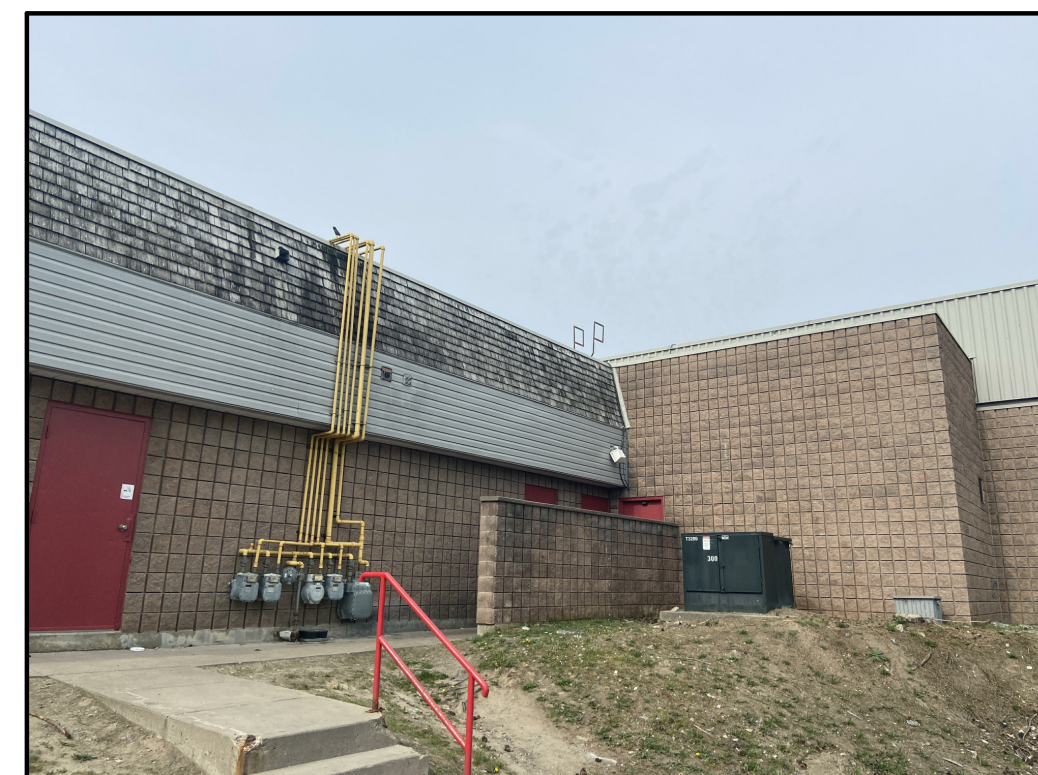
EX. GAS SERVICE LOCATION
