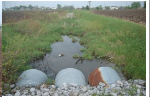
PLATE 22 LOW-LYING WET AREA AND STEEP SLOPE EMBANKMENTS
