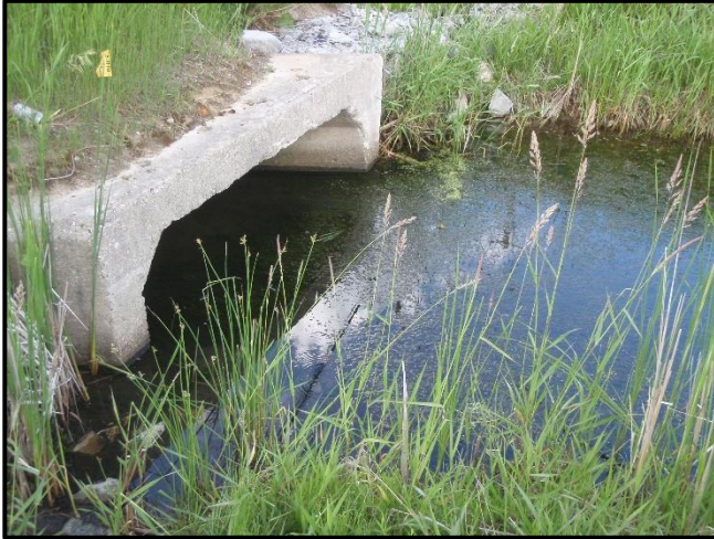
Photograph 1. Location 1. Box culvert at Essa Road, at the downstream extent of the assessed reach. Note the presence of gabion baskets (top of photo). Also note backwatering.
