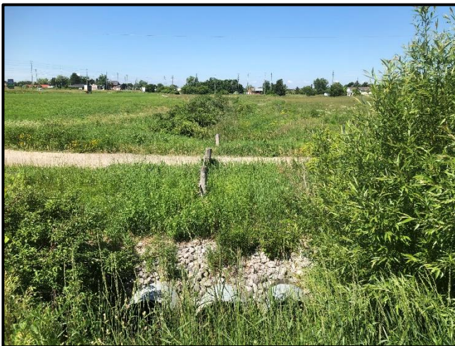
Photograph 7. Location 6. Looking downstream towards the three 1000 mm diameter CSPs at the upstream extent of the reach.
