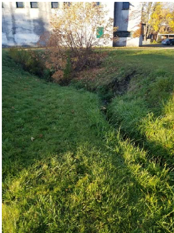
Figure 16 Looking west at the west portion of the open channel of Sophia Creek, October 2022.
