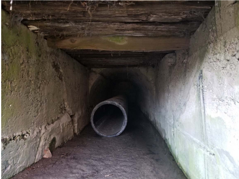
Figure 17 Looking west into the stormwater culvert beneath the west side of the Site, October 2022.
