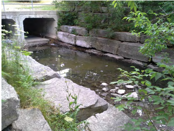
Photograph 13: Perched culvert downstream of Berczk Street (Fisheries Survey Site 10).
